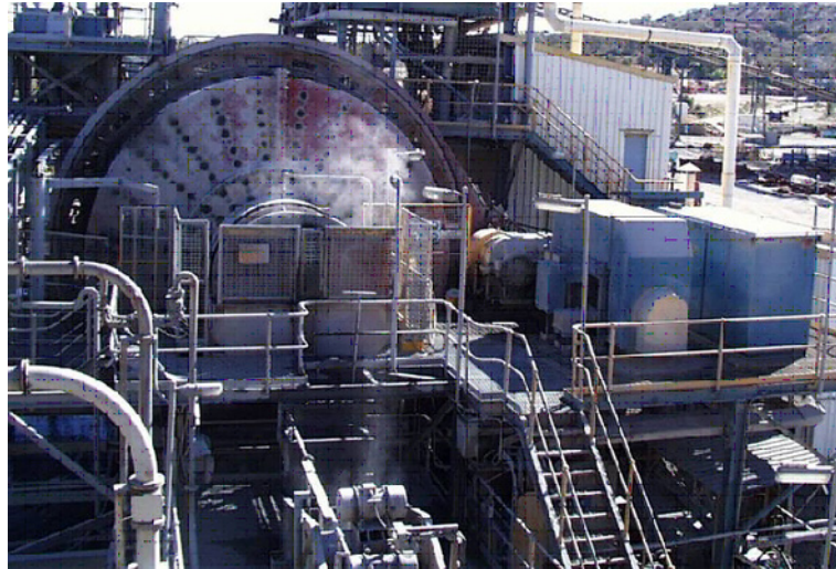
Figure C.1 — Mill drive train misalignment
