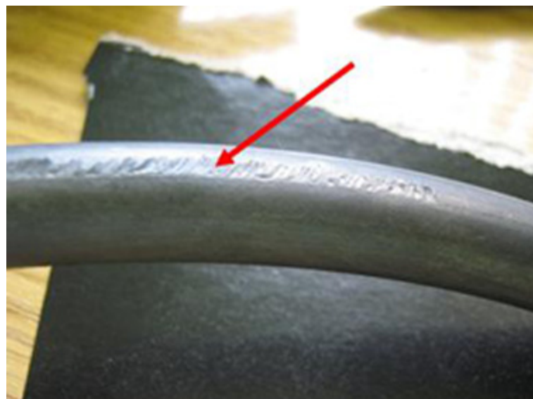
Figure C.2 — Damage caused by abrasive contact with concrete floor
