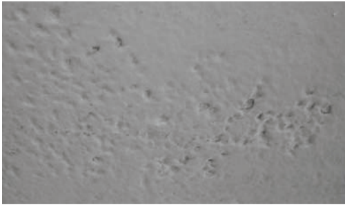
Figure A.15 — Pitting
