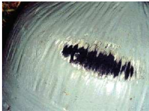
b) Level 2 abrasion damage — Depth of abrasion between 5 % and 15 % of thickness (fully-wrapped cylinder)
