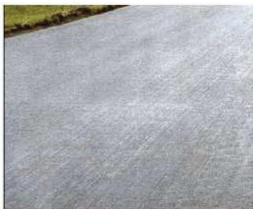
Figure C.4 — Finely milled surface ready for the application of new asphalt concrete top layer (wearing course)
