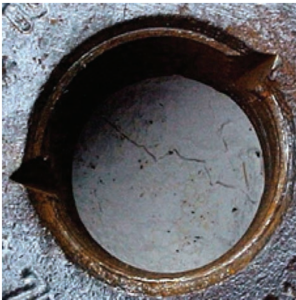
a) Hairline crack without visible sidewalls
