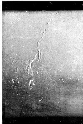
Figure B.2 — Crack
