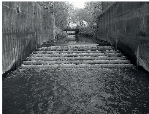
b) Flow condition on a weir with baffles under running condition
