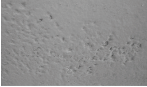
Figure A.15 — Pitting
