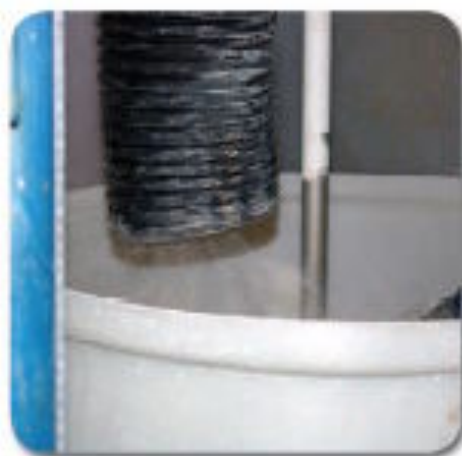
Local exhaust ventilation controlling fugitive emissions during precursor mixing at a primary nanoscale metal oxide production facility.
