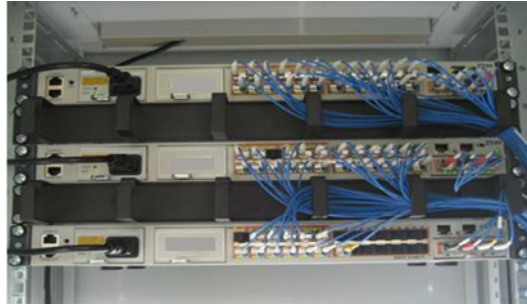
Figure 53 — Fibre switch in a broadband cabinet in a substation
