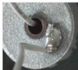
Photo 2: connection on the upper part of the capacitor
