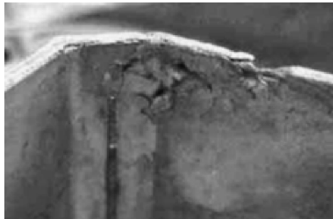
Figure A.30 — Example of incomplete casting
