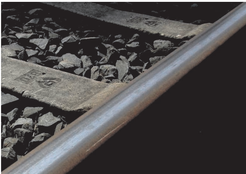
Figure 7 — Visible feature at approximate 0,125 m wavelength present during trolley measurements at Wildenrath over much of the length of the far rail
