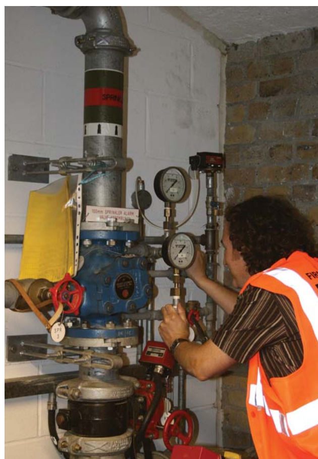
The output of the fire strategy may, for instance, determine that a form of automatic fire suppression, such as a sprinkler system, is most appropriate.
