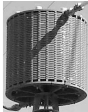
Figure 23 – HV line trap
