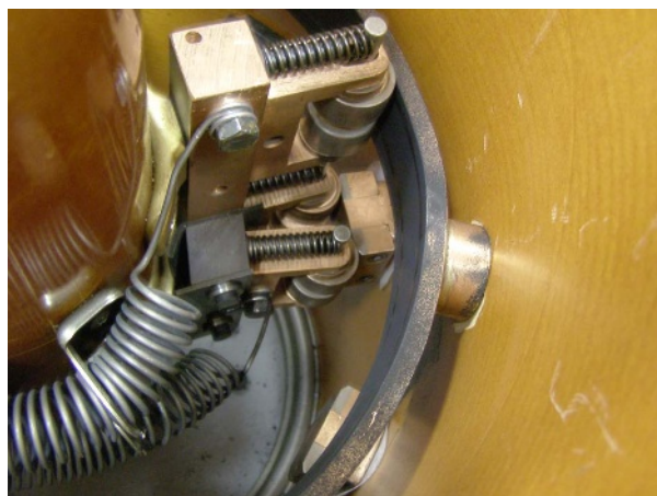
Figure A.47 – Externally strained parts in an on-load tap changer (OLTC)
