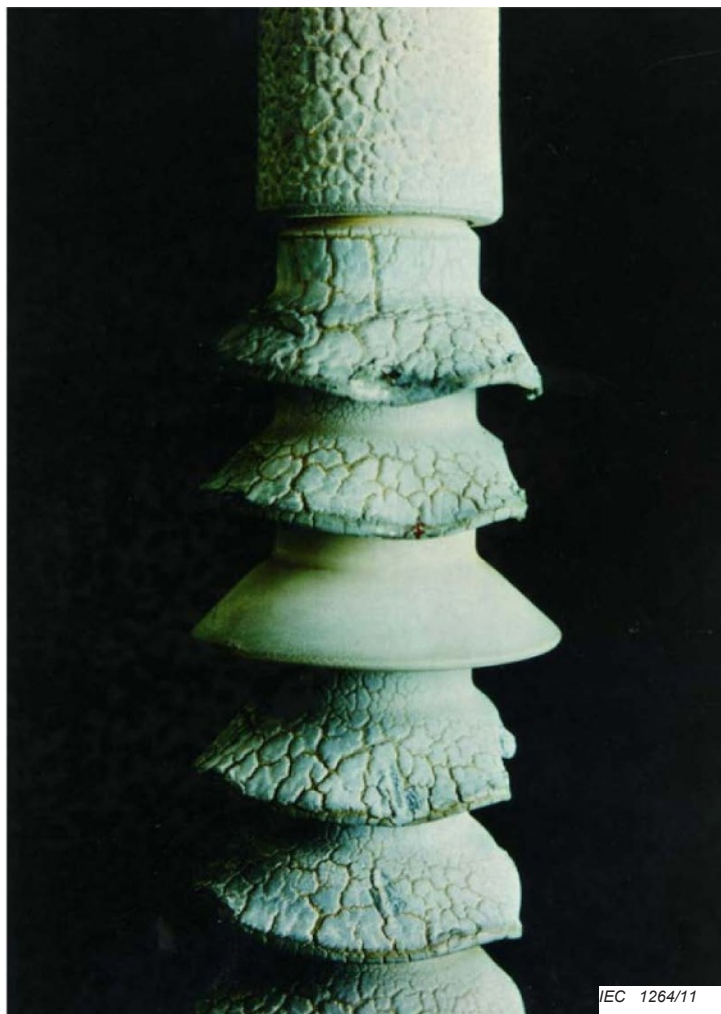
Figure A.27 – EPDM ashing and erosion on fitting
