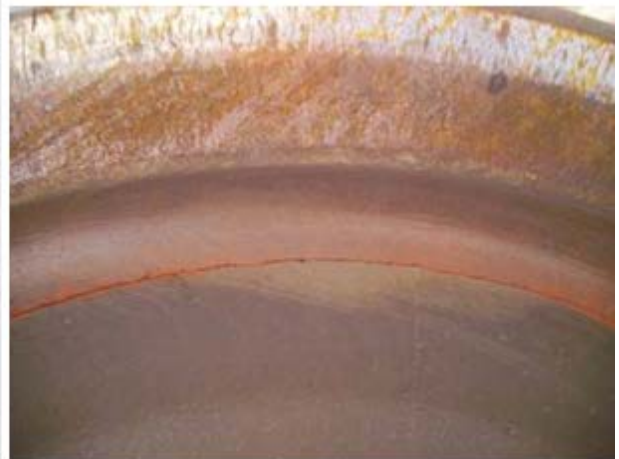
c) — Circumferential cracking below the rim
