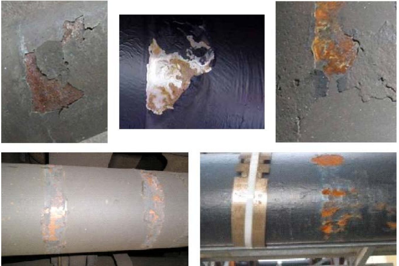
Figure C.34 — Damages of painting/coating
