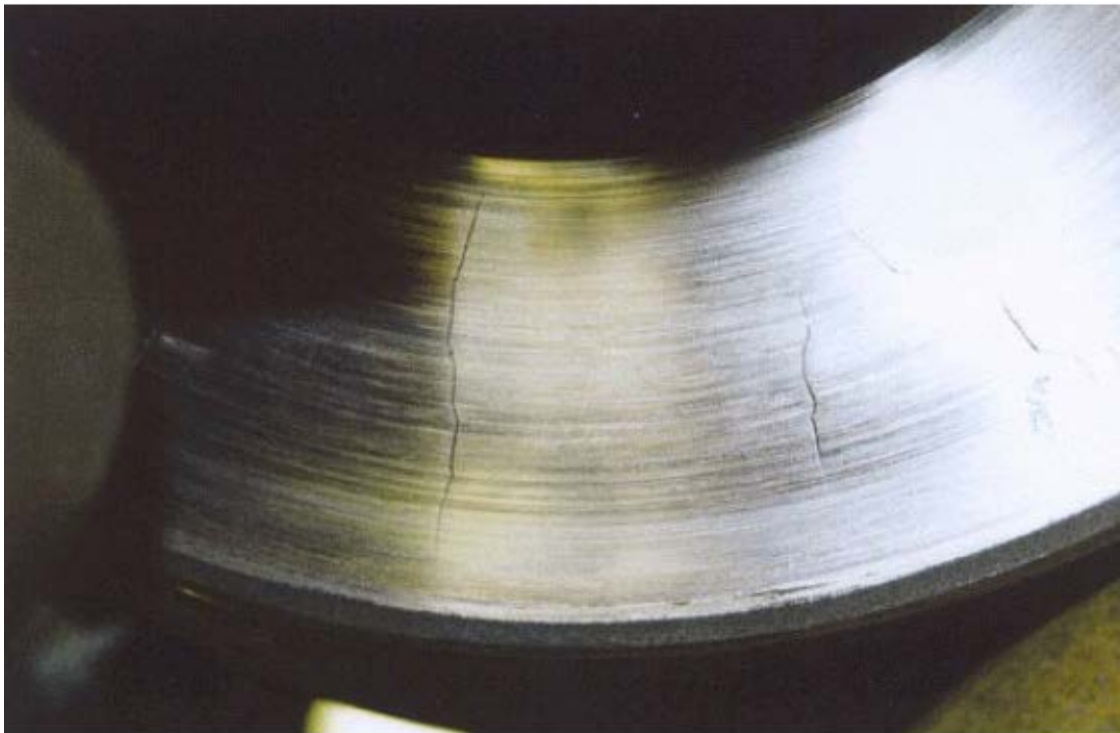
Figure C.31 — Example of defects on the web of a wheel used as a braking surface
