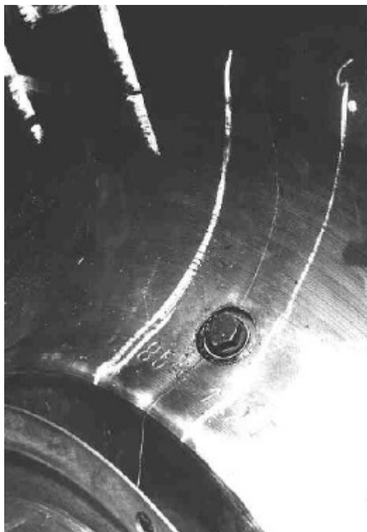
Figure C.29 — Cracks in the hub
