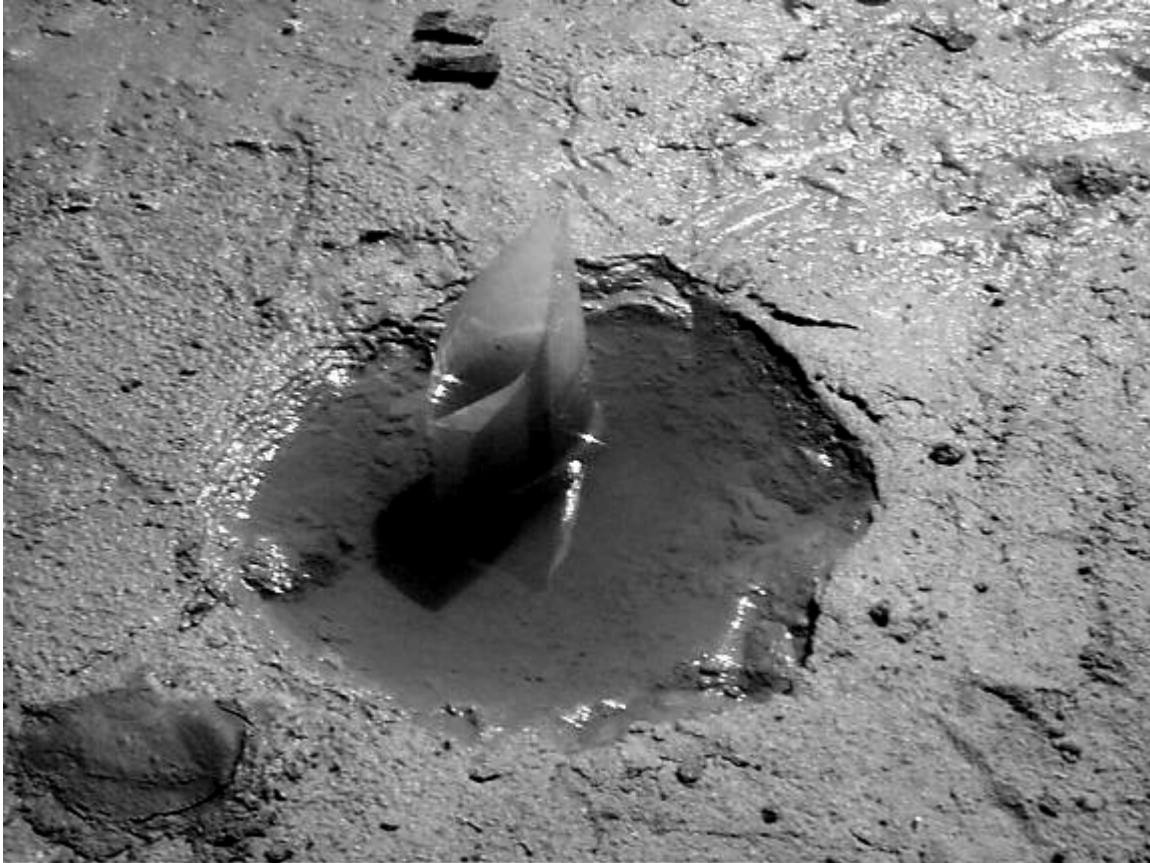
Figure A.12 — Example of drainage blanket of granular material with insufficient permeability, showing water trapped in the drainage blanket, implying backpressure in the drain
