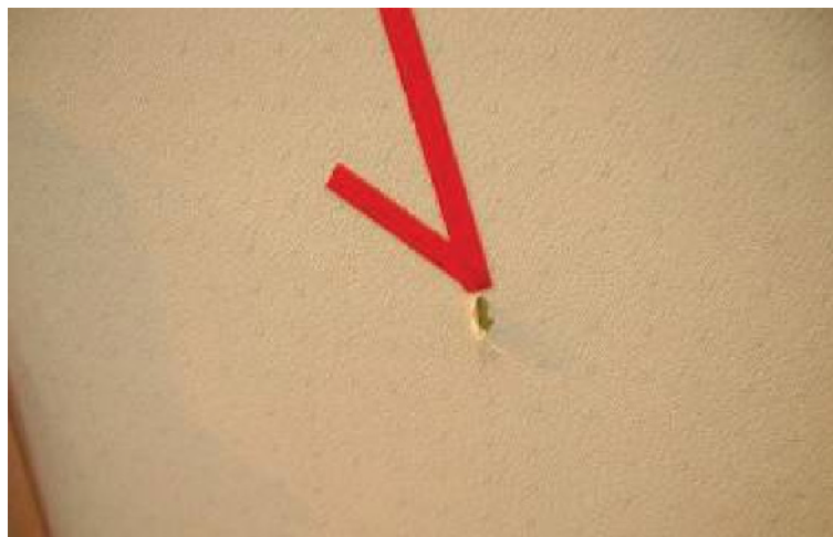
Figure A.1 — Example of a perforation finding
