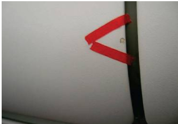
Figure A.37 — Example of a blistering finding
