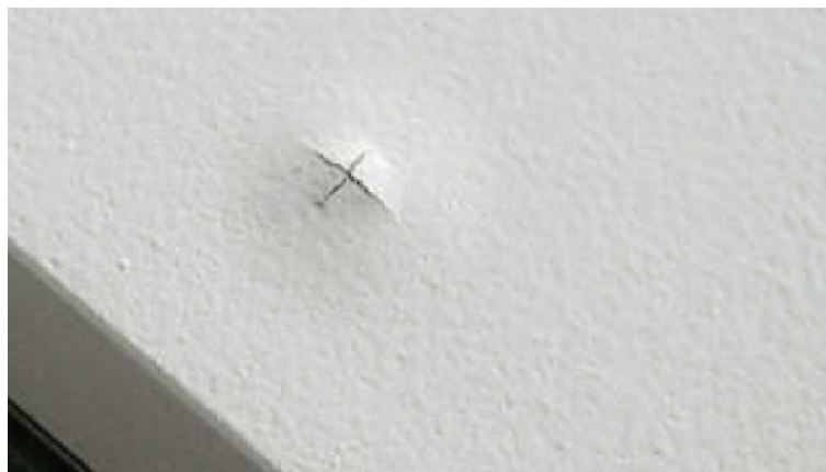
Figure A.27 — Example of a protrusion finding
