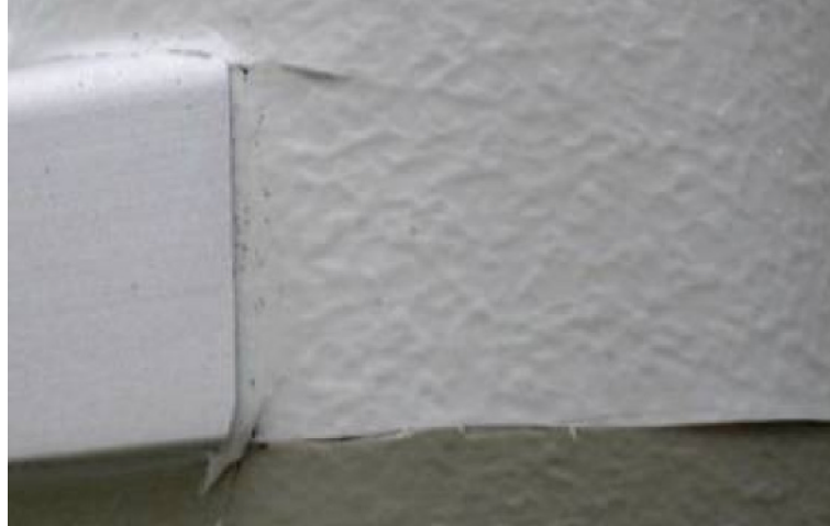
Figure A.19 — Example of a poor trimming finding
