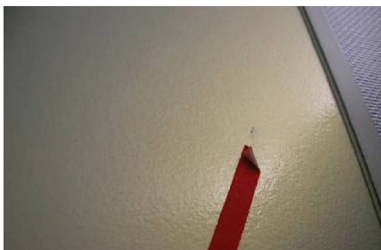
Figure A.4 — Example of a paint defect finding
