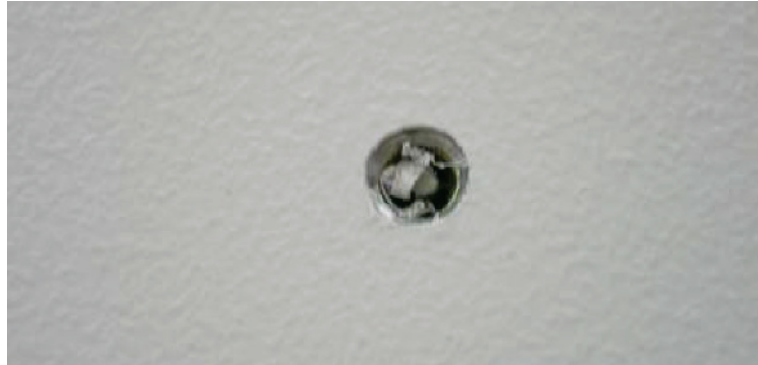
Figure A.34 — Example of a blocked insert finding
