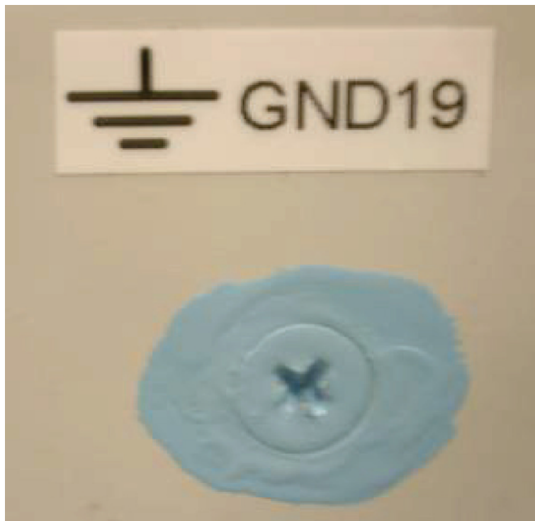
Figure A.30 — Example of a ground screw finding
