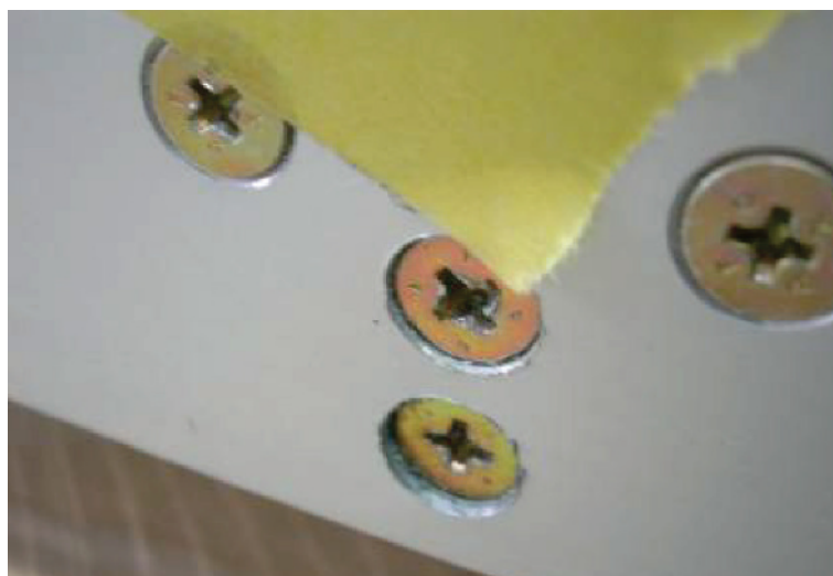
Figure A.31 — Example of a countersink finding
