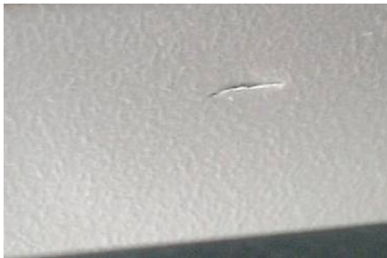
Figure A.2 — Example of a crack finding
