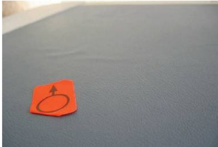
Figure A.7 — Example of a poor adhesion finding
