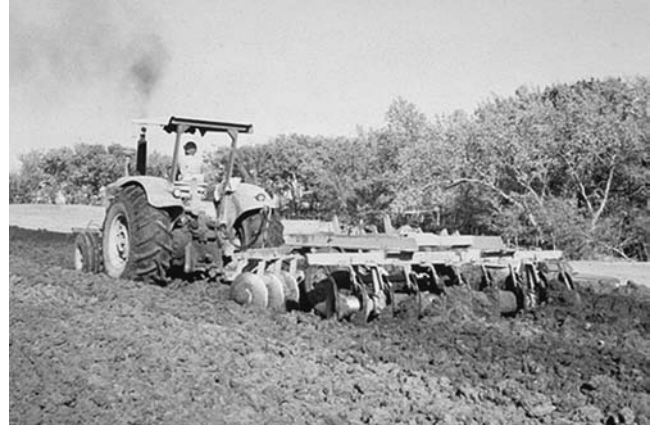
Fig. 4—Disking earth fill to break up soil clods and/or incorporate water. The disking may also be used to dry out wet soil.
