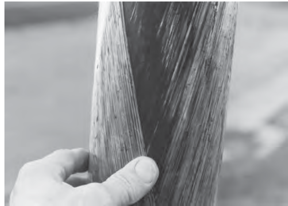
Fig. 6-18—Matrix erosion on a composite light post used outdoors.
