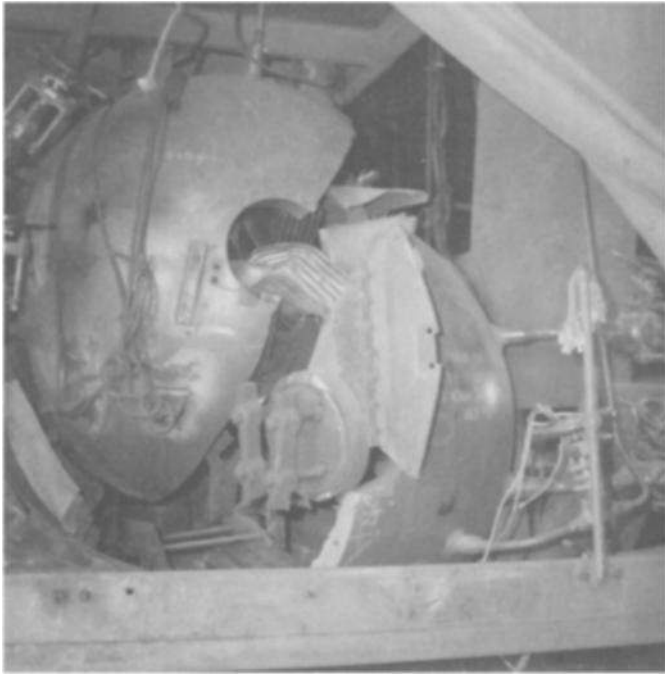
Fig. 10.2 —Brittle failure of a fabricated high-pressure water-tube boiler drum during initial hydrostatic test. Origin was a large undetected crack at the toe of a nozzle weld that occurred during the post weld heat treatment cycle.
