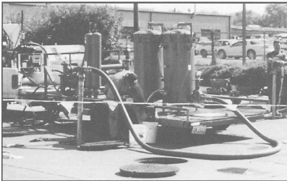
FIG. 2—Recirculating underground storage tank cleaning system. Suction riser from tank is at far right. Suction line (in background) leads to API separator alongside power pack set on truck (left). Fuel then flows through first-stage housing with coalescer media (center-left) and particulate final filter (center-right) before flowing through return riser (foreground-left). Photo courtesy of Fuel Quality Services, Inc.
