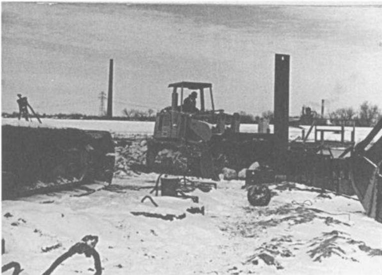
FIG. 18.3 Sand piled on cofferdam cells and the front-end loader used to push it overboard.
