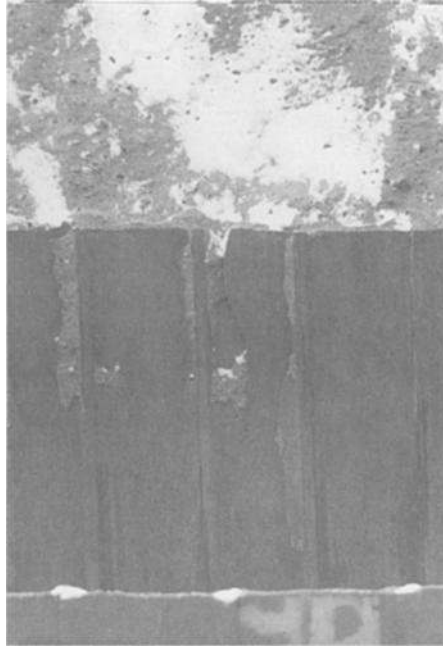
FIG. 18.8 Nonpropagating crack in sheet pile.
