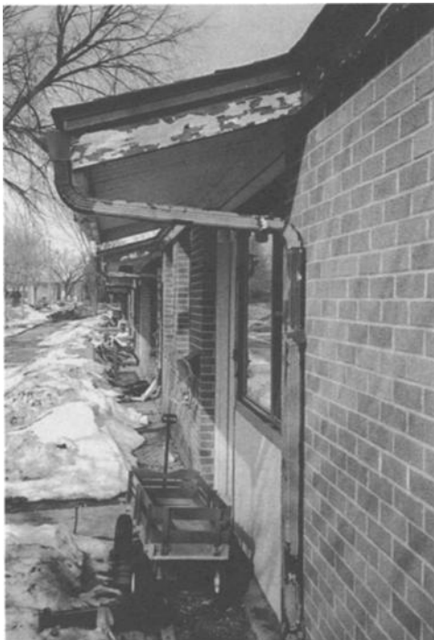
Figure 1.1: This married student housing facility is a good candidate for a Lead Hazard Management Program
