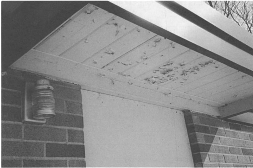
Figure 11.2: Leaded paint peeling from soffit before control.
