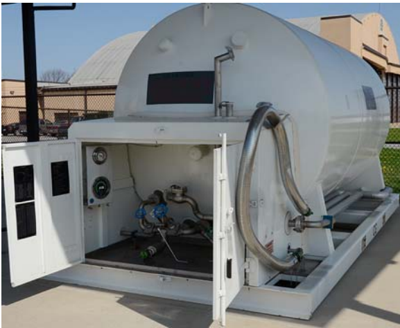
FIG. 1 Skid-Mounted Cryogenic Oxygen Storage Image courtesy of Essex Industries
