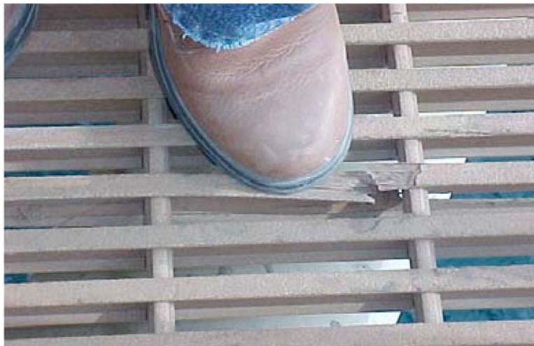
FIG. X2.1 Broken Bearing Bar; Trip Hazard
