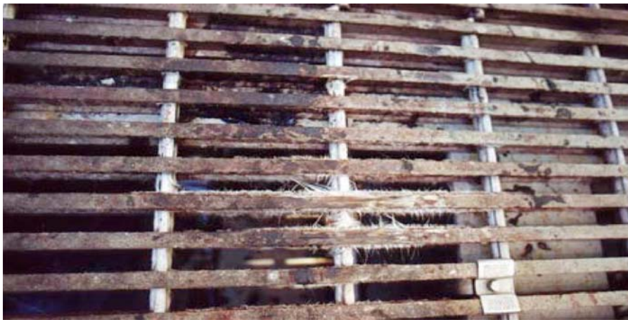
FIG. X1.11 Damage to FRP Gratings from Chemical Exposure
