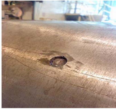
FIG. X2.2 (Reference Fig. X2.1. One circumferential crack on the ID was ~6 mm [ \frac{1}{4} in.] long. The other crack on the OD was ~12 mm [ \frac{1}{2} in.] long.
