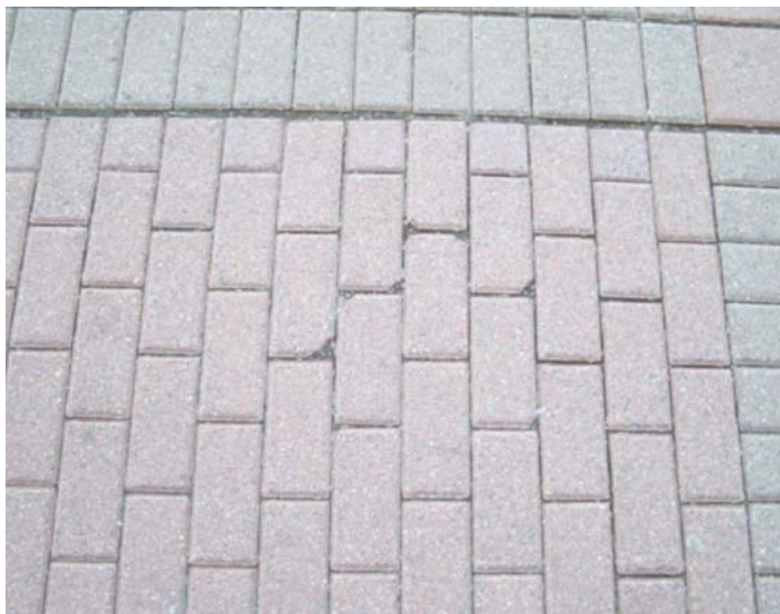
FIG. X1.1 Low Severity Damaged Pavers
