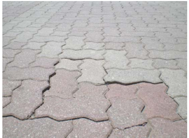
FIG. X1.14 Medium Severity Faulting
