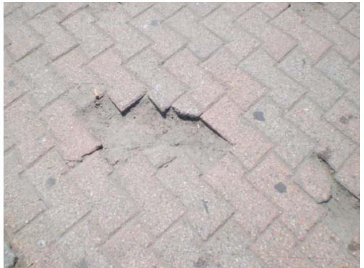
FIG. X1.26 Medium Severity Missing Pavers
