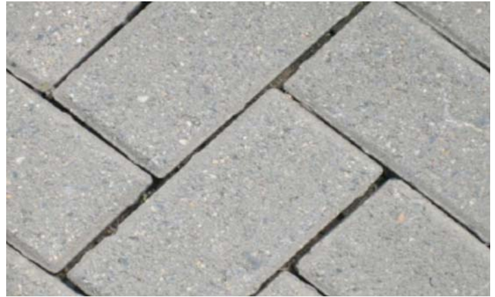
FIG. X1.22 Low Severity Joint Sand Loss
