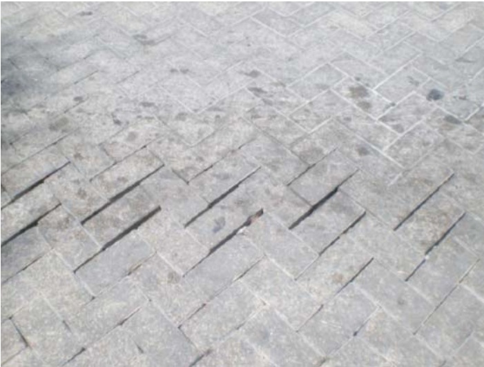
FIG. X1.12 High Severity Excessive Joint Width (greater than 1/2 in. (13 mm))
