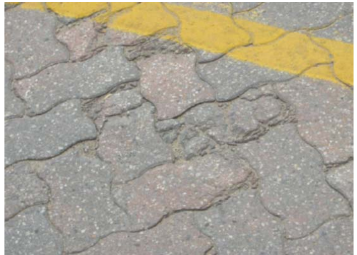
FIG. X1.2 Medium Severity Damaged Pavers
