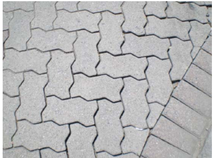
FIG. X1.11 Medium Severity Excessive Joint Width
