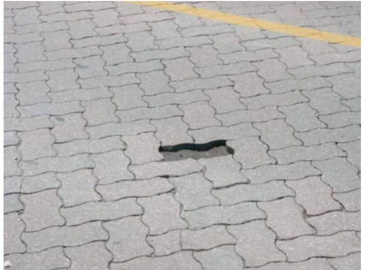
FIG. X1.25 Low Severity Missing Pavers
