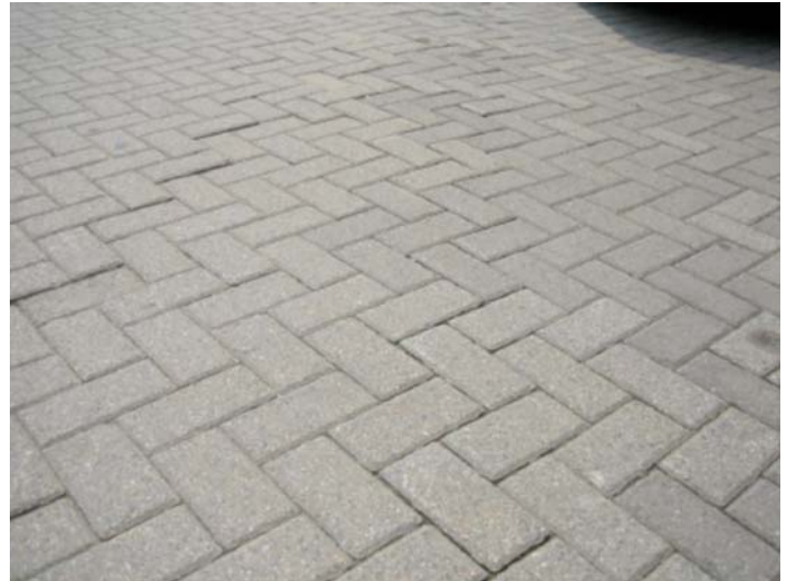
FIG. X1.13 Low Severity Faulting
