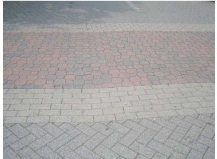
FIG. X1.4 Low Severity Depression
