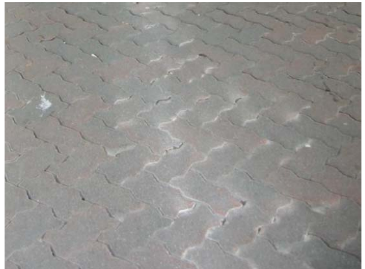
FIG. X1.23 Medium Severity Joint Sand Loss
