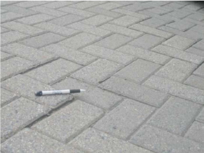
FIG. X1.15 High Severity Faulting
