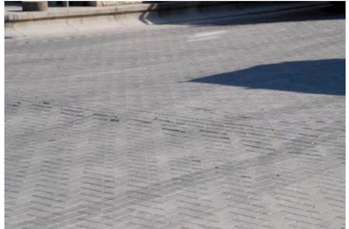
FIG. X1.16 Low Severity Heave
