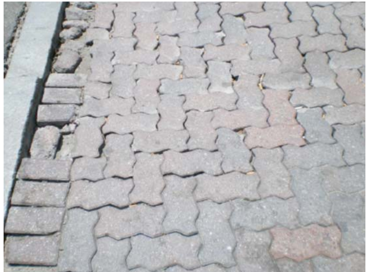
FIG. X1.8 Medium Severity Loss of Edge Restraint
