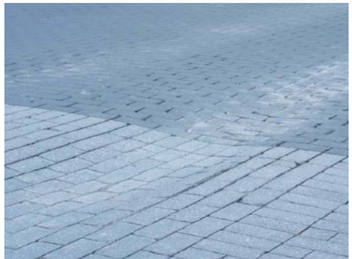
FIG. X1.32 Medium Severity Rutting
