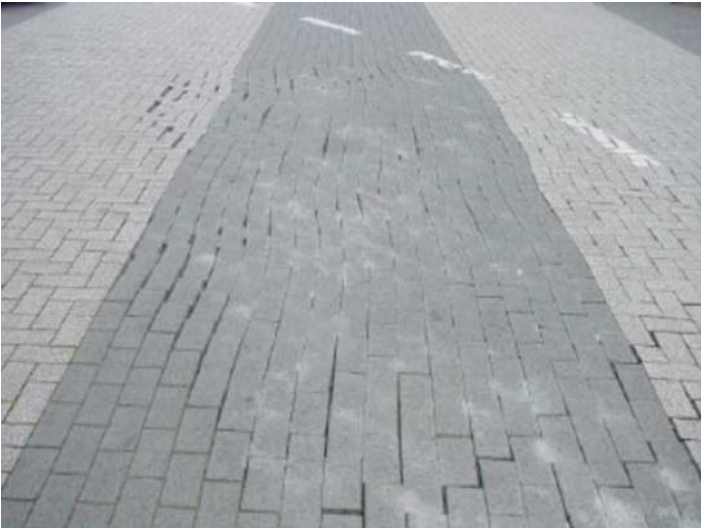
FIG. X1.9 High Severity Loss of Edge Restraint
