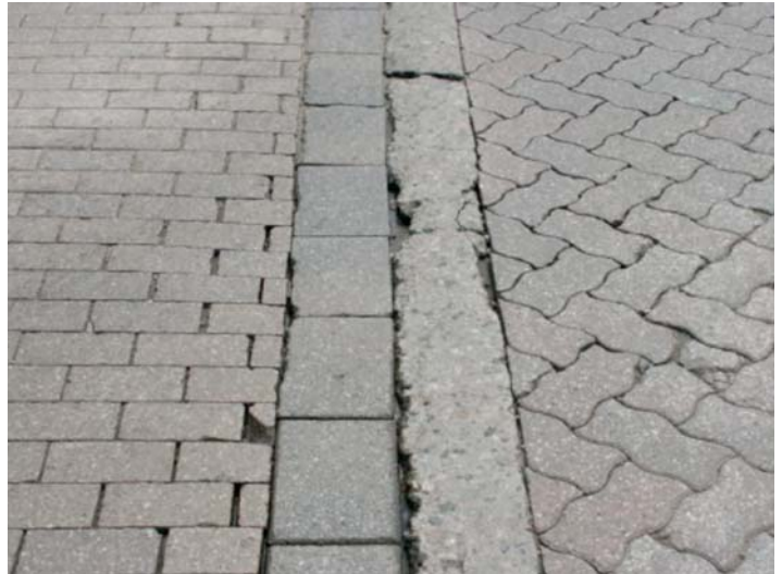
FIG. X1.7 Low Severity Loss of Edge Restraint
