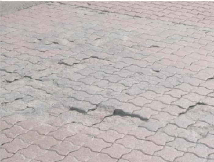
FIG. X1.3 High Severity Damaged Pavers
