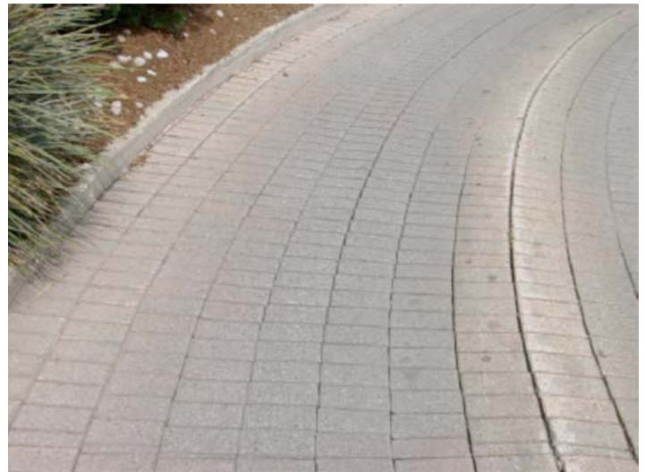
FIG. X1.31 Low Severity Rutting
