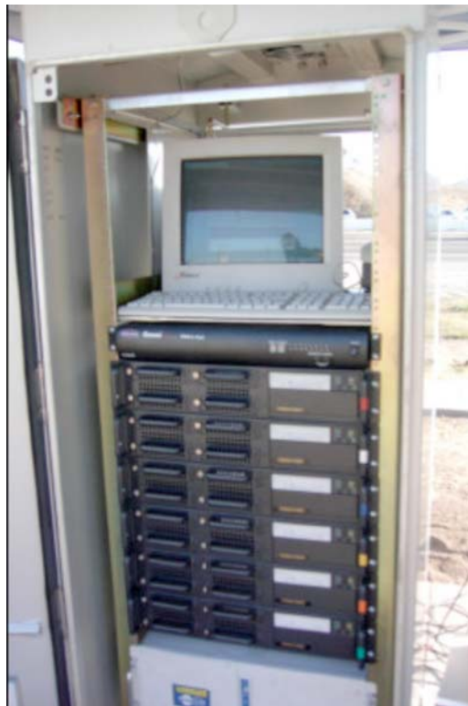
FIG. X2.2 V 2 DVS Data Acquisition Computers in Type 334C Cabinet
