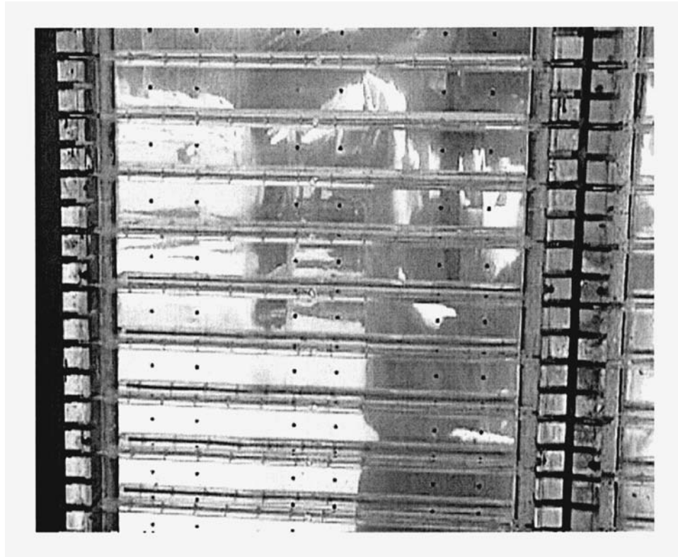
FIG. 15 Close-up of Lamps and Lamp Panel
