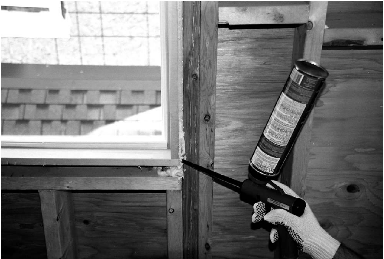
FIG. A1.1 Application of Aerosol Foam Sealant (Type A Material) In Cavity Between Window Frame and Rough Opening
