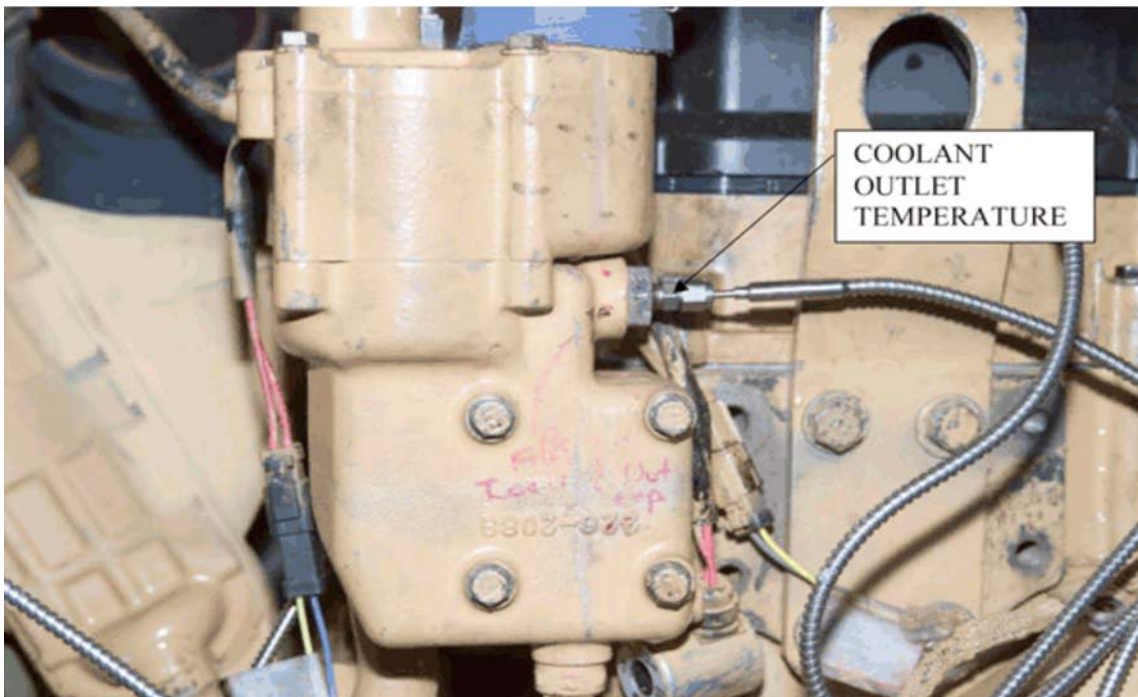
FIG. A5.13 Coolant-Outlet Temperature
