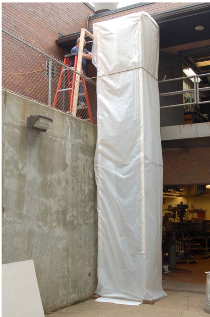
FIG. 1 Dry Fall Evaluation Enclosure with Plastic Sheeting (Note—Base is heightened using 1.5 in. wooden blocks.)
