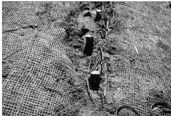
NOTE 1—A rolled erosion control product was also used in this example FIG. 3 Photograph of Typical Complete Live Fascine Construction
