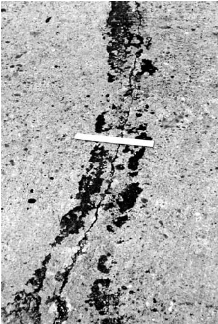
FIG. X2.22 Low-Severity Linear Cracking
