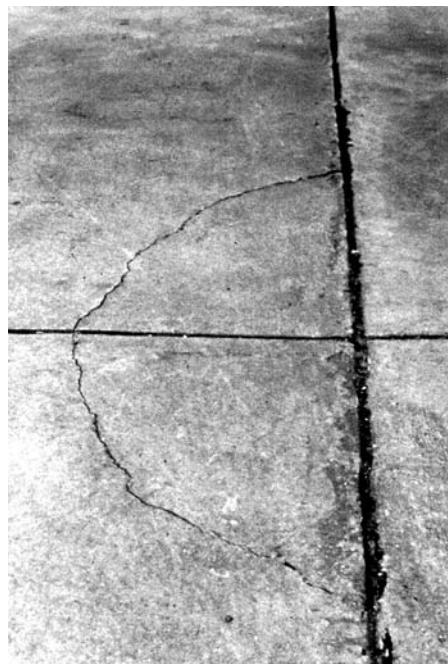
FIG. X2.4 Low-Severity Corner Break
