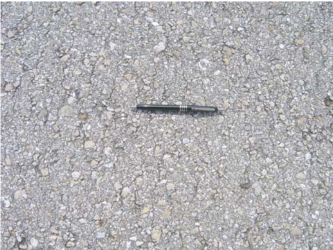
FIG. X1.53 Low-Severity Weathering (Surface Wear)
