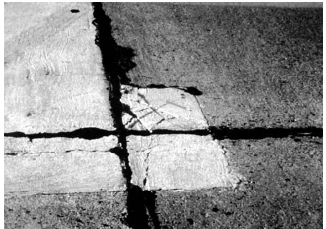
FIG. X2.29 Medium-Severity Patching, Small
