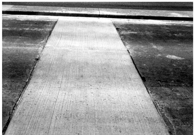
FIG. X2.25 Low-Severity Patching, Large and Utility Cuts
