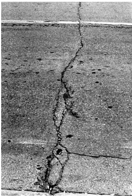
FIG. X1.23 Medium-Severity Joint Reflection Cracking
