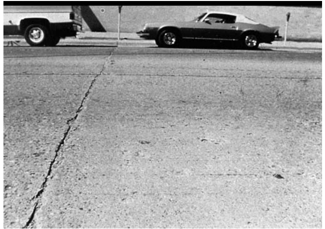
FIG. X2.48 Low-Severity Spalling, Joint
