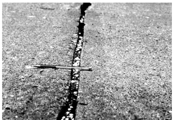
FIG. X2.18 High-Severity Joint Seal Damage
