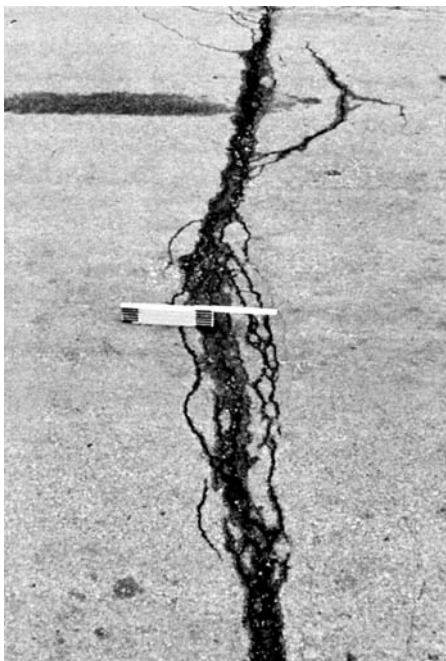
FIG. X1.24 High-Severity Joint Reflection Cracking
