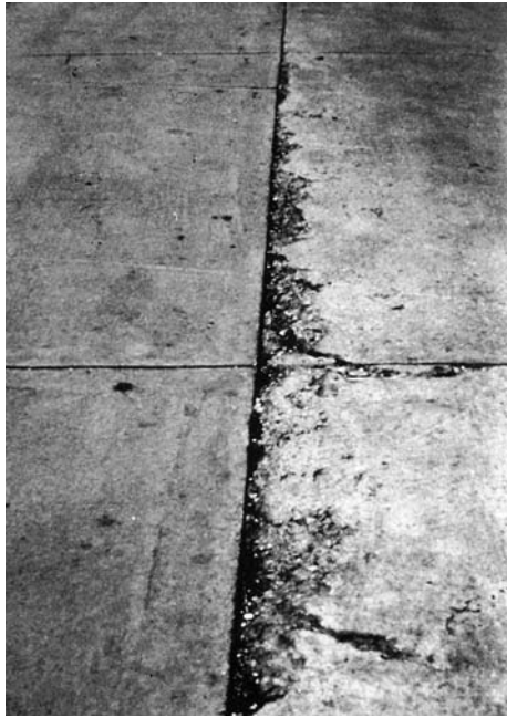
FIG. X2.49 Medium-Severity Spalling, Joint
