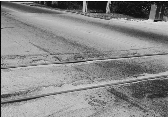
FIG. X1.39 Medium-Severity Railroad Crossing
