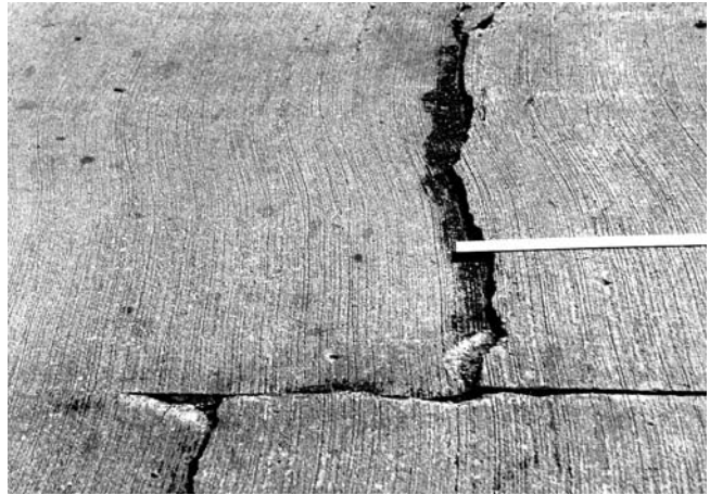
FIG. X2.24 High-Severity Linear Cracking
