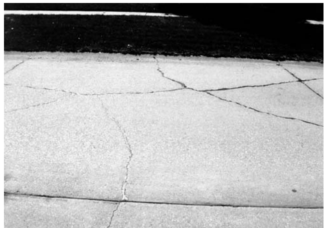
FIG. X2.8 Medium-Severity Divided Slab
