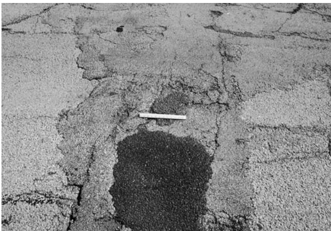
FIG. X1.33 High-Severity Patching and Utility Cut Patching
