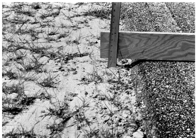
FIG. X1.25 Low-Severity Lane/Shoulder Drop-Off
