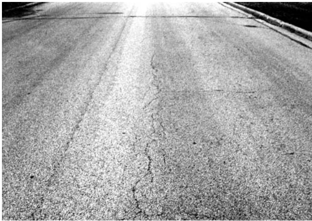
FIG. X1.1 Low-Severity Alligator Cracking
