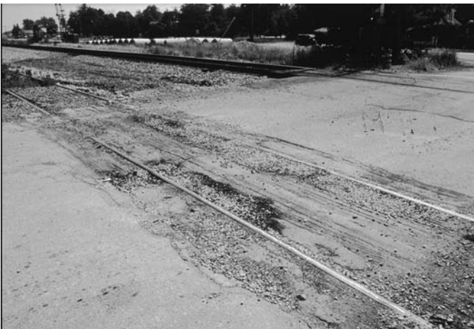
FIG. X1.40 High-Severity Railroad Crossing
