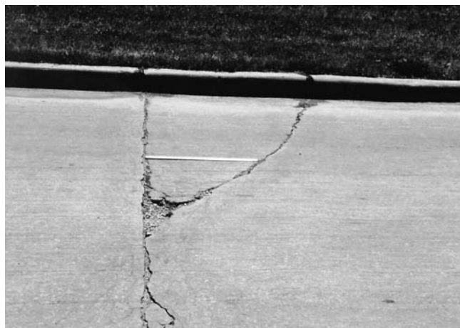
FIG. X2.5 Medium-Severity Corner Break
