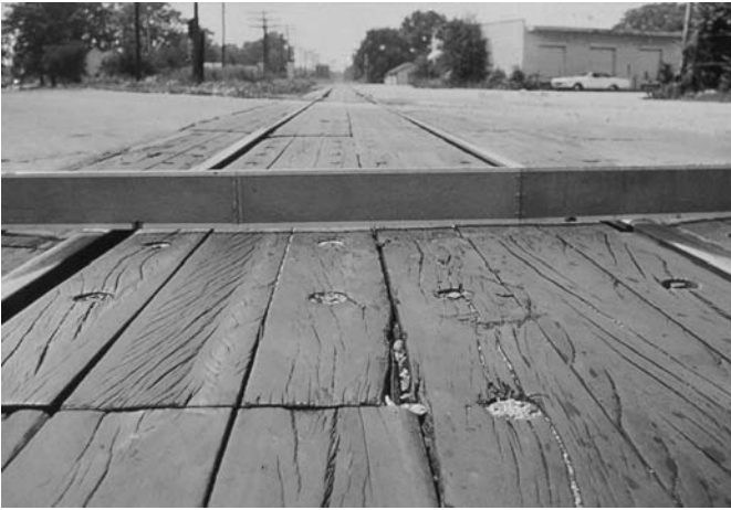
FIG. X1.38 Low-Severity Railroad Crossing
