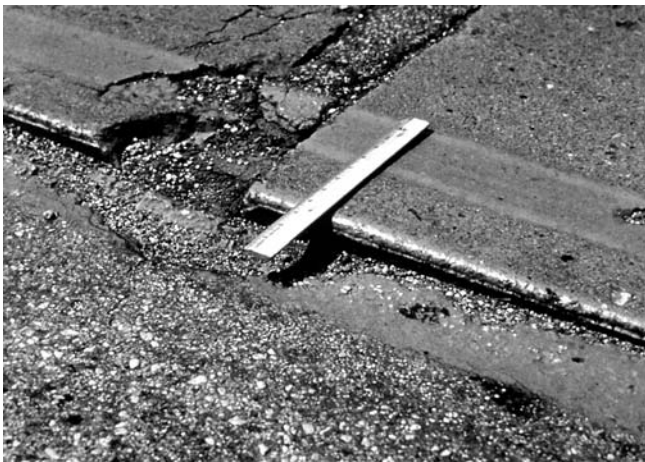
FIG. X2.19 Low-Severity Lane/Shoulder Drop-Off
