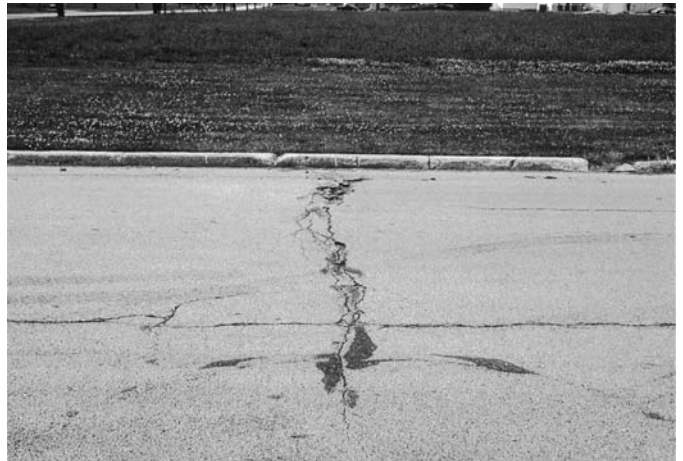
FIG. X1.30 High-Severity Longitudinal and Transverse Cracking
