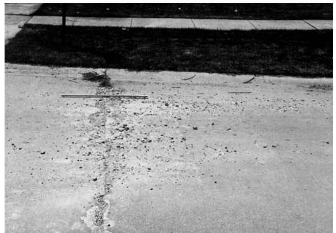
FIG. X2.1 Low Severity Blowup/Buckling
