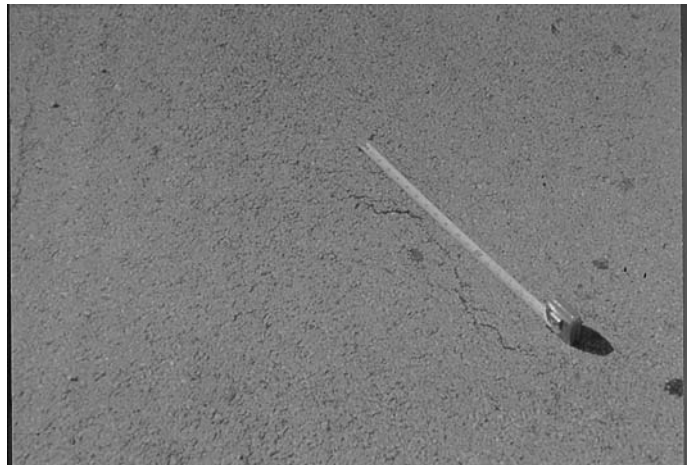
FIG. X1.47 Low-Severity Slippage Cracking
