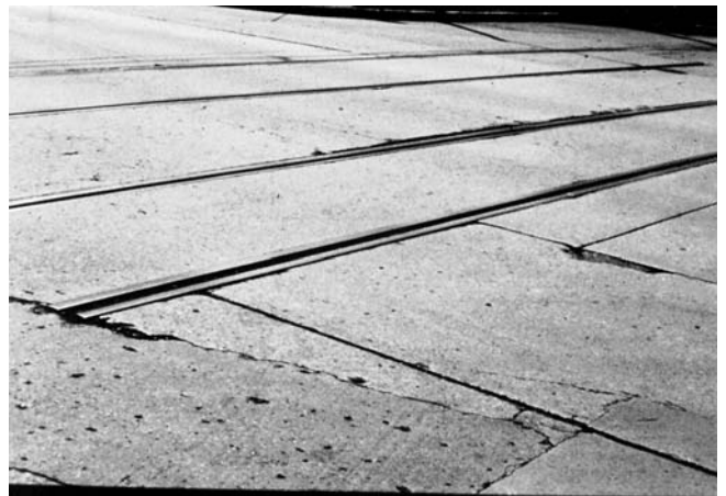
FIG. X2.38 Low-Severity Railroad Crossing
