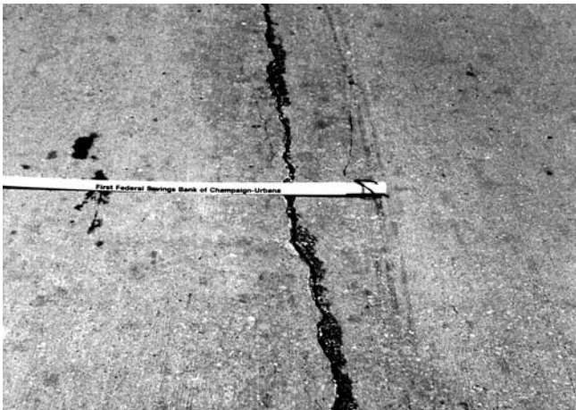
FIG. X2.23 Medium-Severity Linear Cracking
