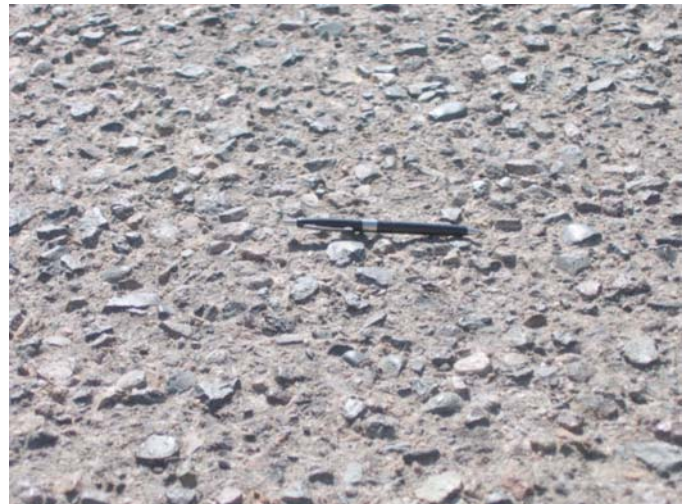
FIG. X1.55 High-Severity Weathering (Surface Wear)
