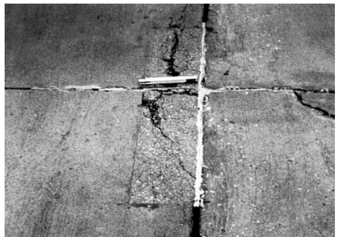
FIG. X2.30 High-Severity Patching, Small
