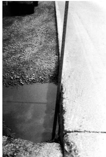
FIG. X2.21 High-Severity Lane/Shoulder Drop-Off
