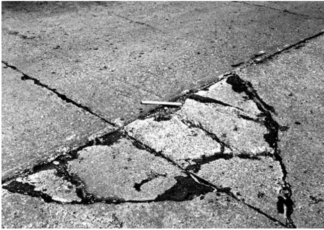
FIG. X2.6 High-Severity Corner Break
