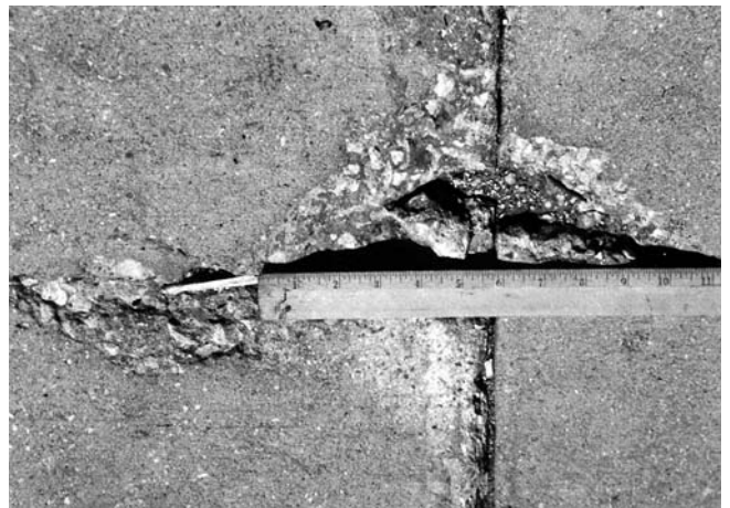
FIG. X2.46 Medium-Severity Spalling, Corner
