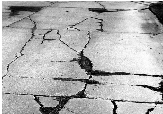
FIG. X2.9 High-Severity Divided Slab
