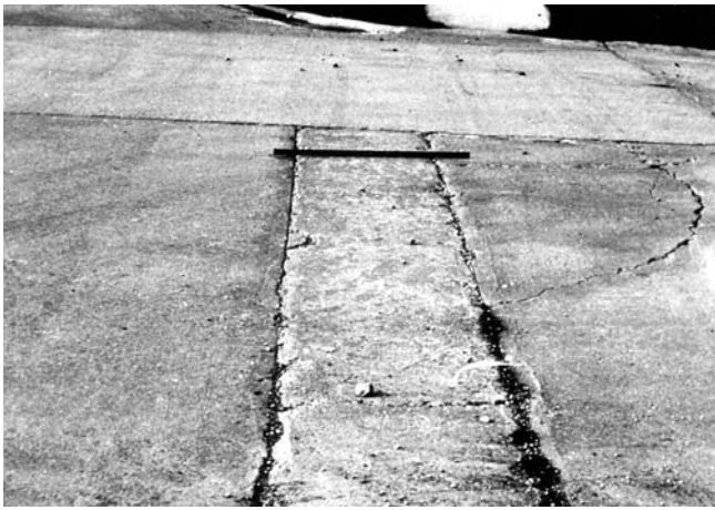
FIG. X2.26 Medium-Severity Patching, Large and Utility Cuts
