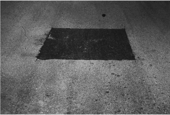
FIG. X1.31 Low-Severity Patching and Utility Cut Patching
