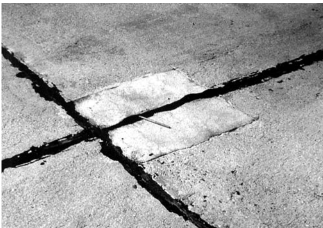
FIG. X2.28 Low-Severity Patching, Small
