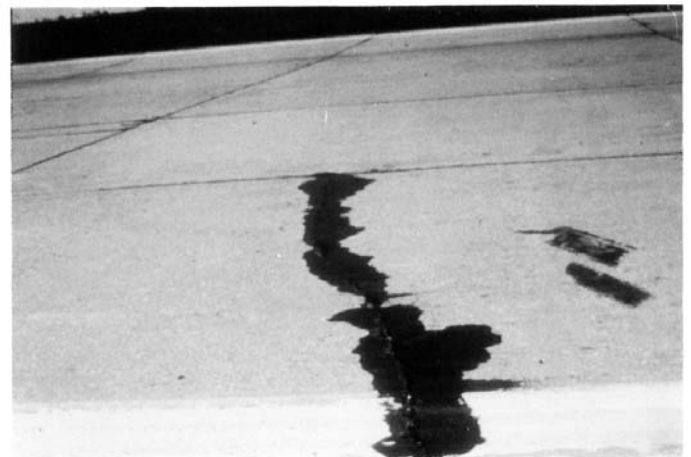
FIG. X2.13 Medium-Severity Transverse Crack
