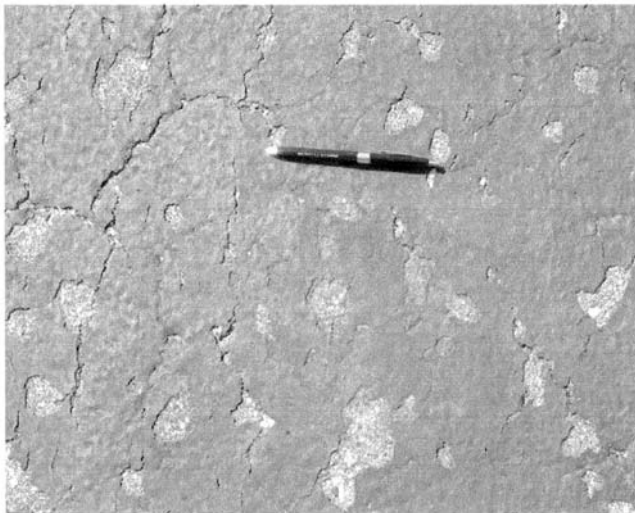
FIG. X1.60 High-Severity Raveling, Cold Tar
