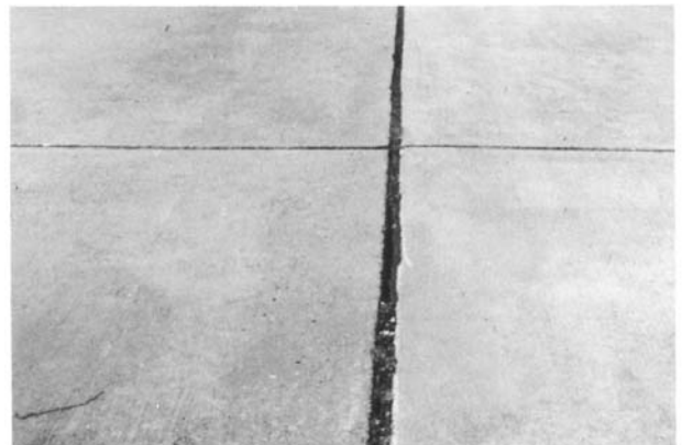
FIG. X2.26 High-Severity Joint Seal Damage (Complete Loss of Sealant; Joint is Filled with Incompressible Material)
