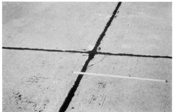
FIG. X2.68 Low-Severity Corner Spall
