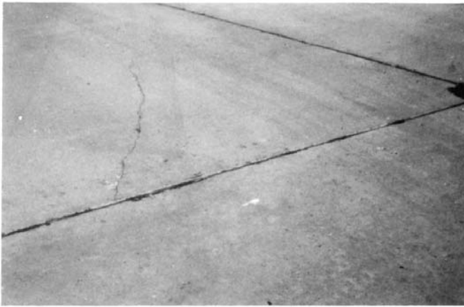
FIG. X2.11 Low-Severity Diagonal Crack
