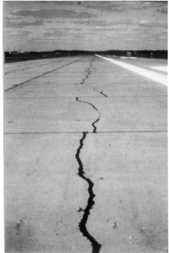
FIG. X2.12 Medium-Severity Longitudinal Crack
