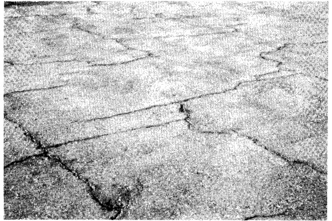
FIG. X1.17 Medium-Severity Block Cracking
