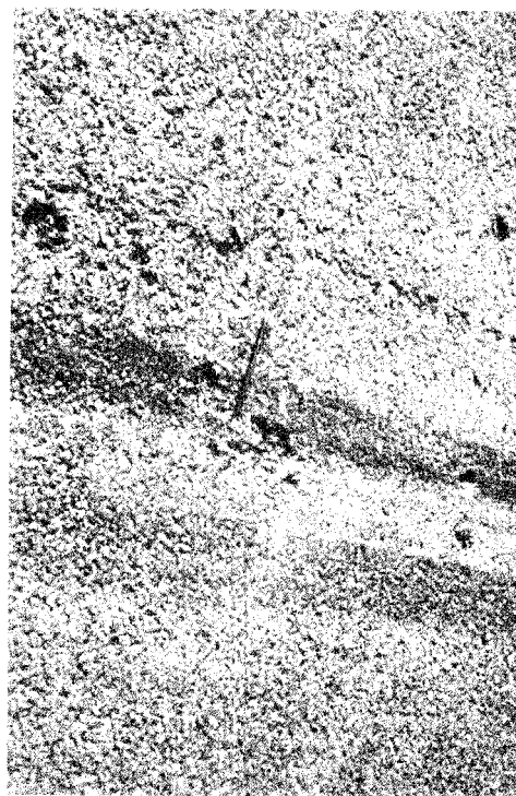
FIG. X1.65 High-Severity Raveling on a Porous Friction Course Surface
