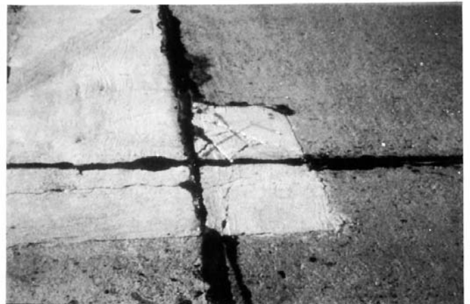
FIG. X2.31 Medium-Severity Small Patch
