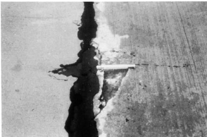
FIG. X2.65 Medium-Severity Joint Spall
