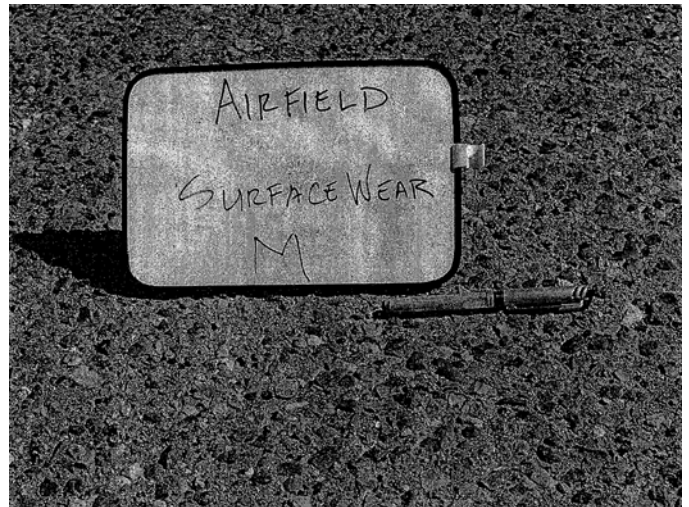
FIG. X1.80 Medium-Severity Weathering (Surface Wear)
