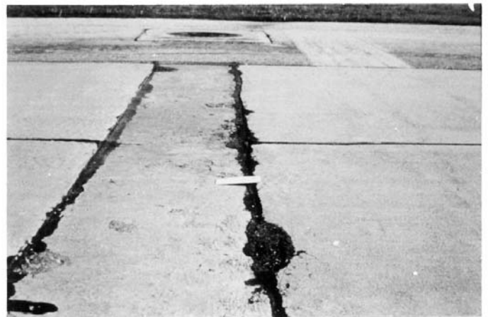
FIG. X2.36 Medium-Severity Utility Cut
