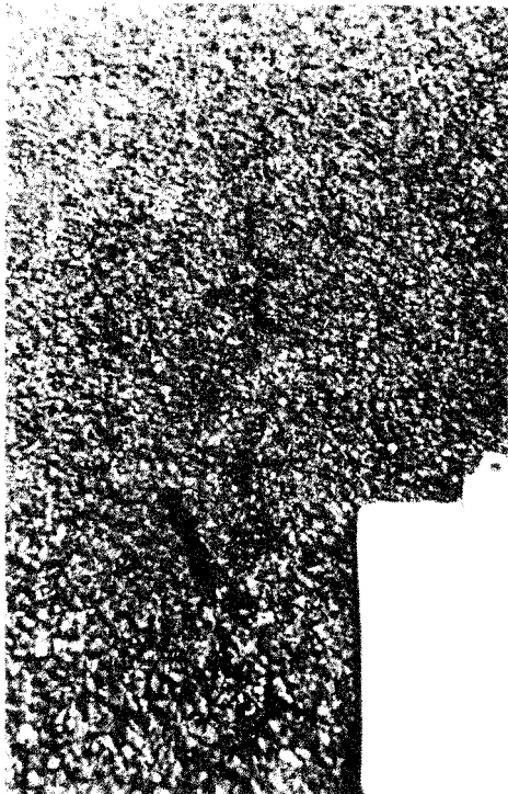
FIG. X1.44 Medium-Severity Crack in Porous Friction Course
