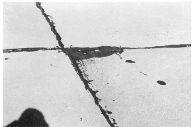
NOTE 1—Slab is beginning to break up near corner. FIG. X2.19 Low-Severity "D" Cracking Approaching Medium Severity
