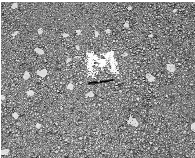
FIG. X1.56 Medium-Severity Raveling, Dense Mix
