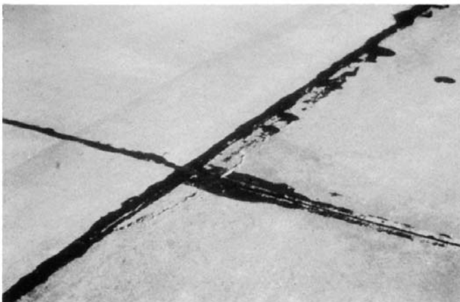
FIG. X2.69 Low-Severity Corner Spall
