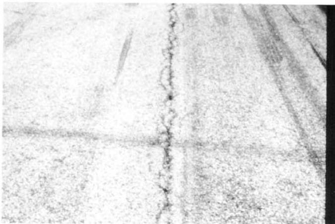
FIG. X1.39 Medium-Severity Longitudinal Construction Joint Crack
