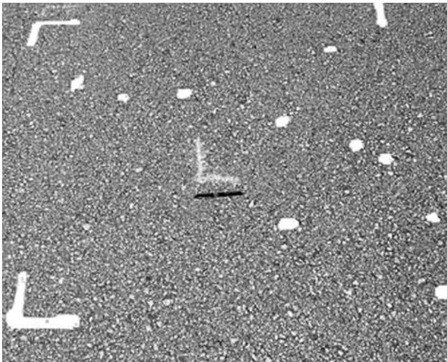
FIG. X1.55 Low-Severity Raveling, Dense Mix
