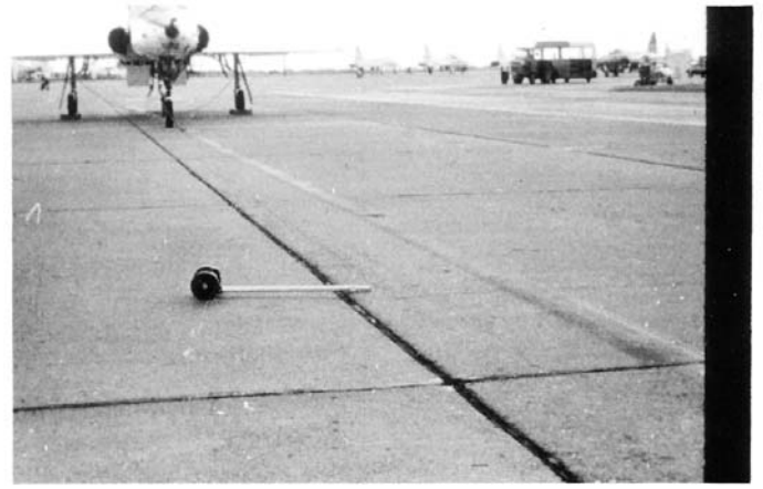
FIG. X2.49 Low-Severity Settlement on Apron
