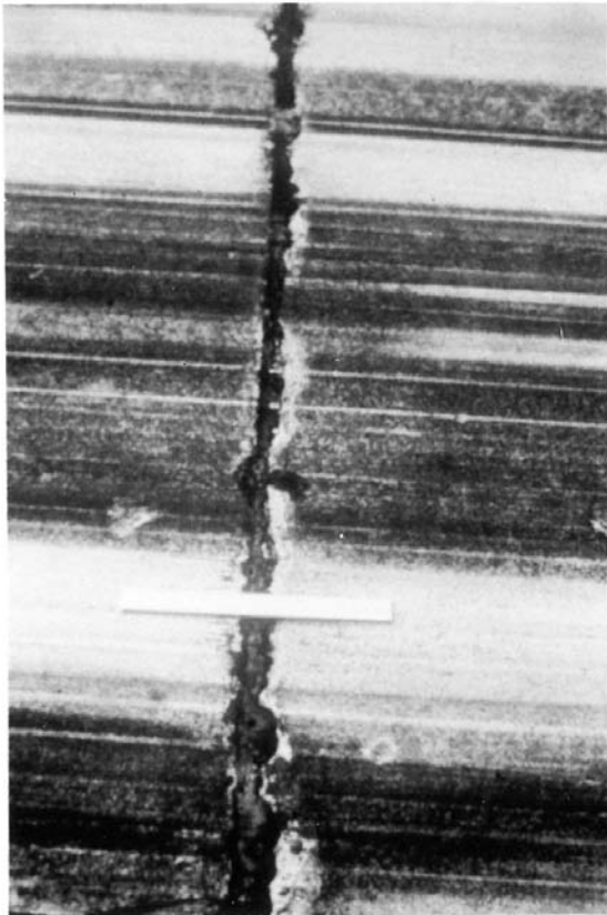
FIG. X2.61 Low-Severity Joint Spalling (If the Frayed Area was Less Than 2 ft (0.6 m) Long it Would not be Counted)
