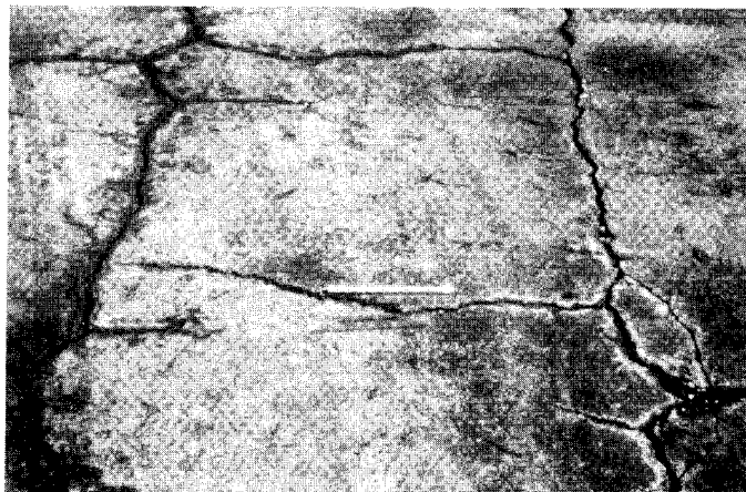
FIG. X1.16 Medium-Severity Block Cracking
