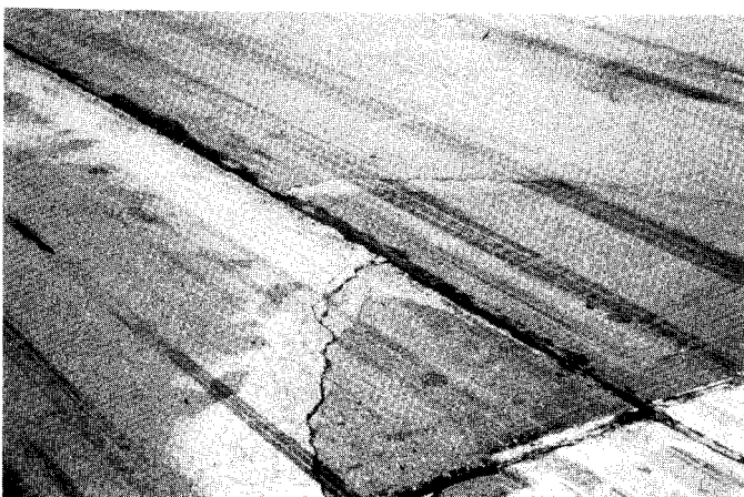
FIG. X2.7 Medium-Severity Corner Break
