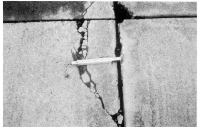
FIG. X2.71 Medium-Severity Corner Spall
