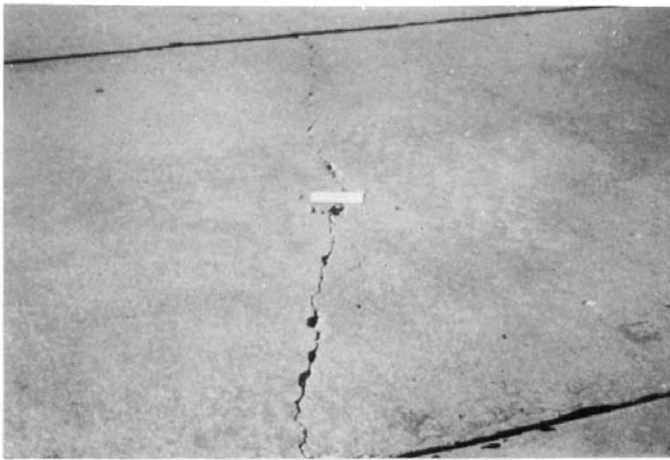
FIG. X2.14 Medium-Severity Transverse Crack
