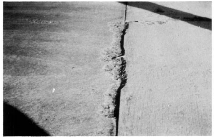
FIG. X2.67 High-Severity Joint Spall
