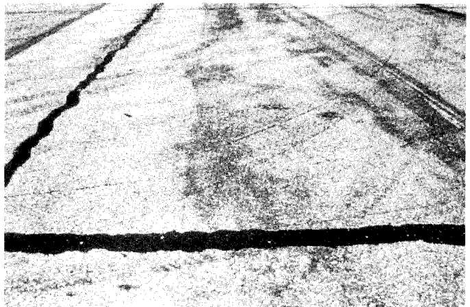
FIG. X1.31 Low-Severity Joint Reflection Cracking, Filled Crack
