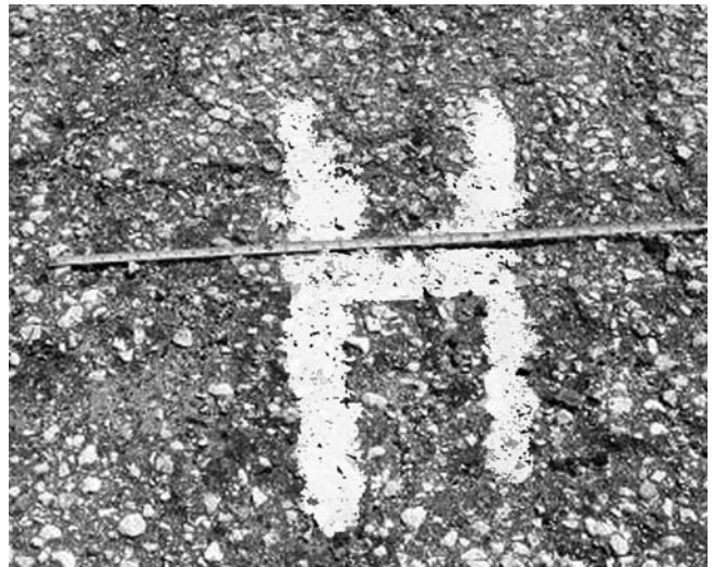
FIG. X1.57 High-Severity Raveling, Dense Mix
