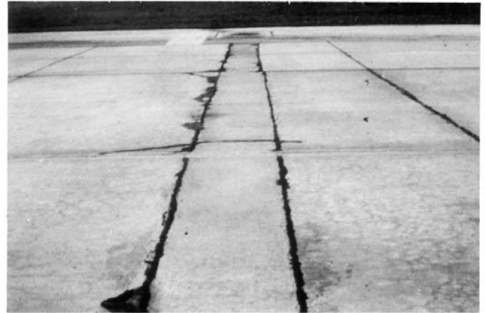
FIG. X2.35 Low-Severity Utility Cut
