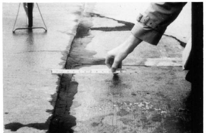
FIG. X2.50 Medium-Severity Settlement on Apron (> \frac{1}{2} in. (13 mm))
