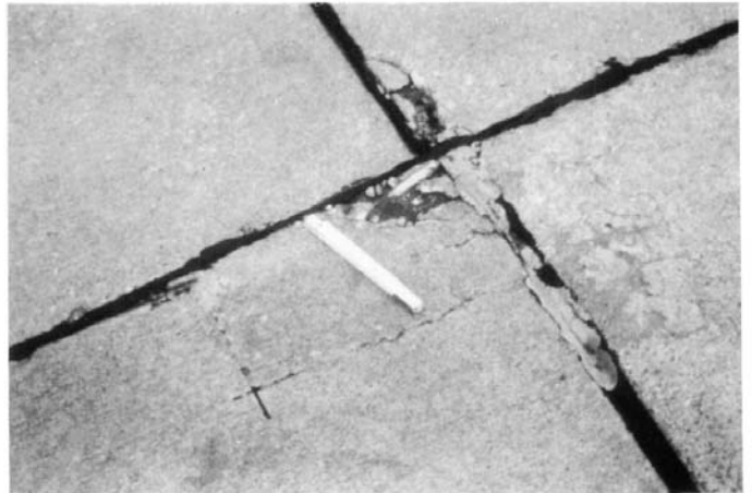
FIG. X2.30 Medium-Severity Small Patch
