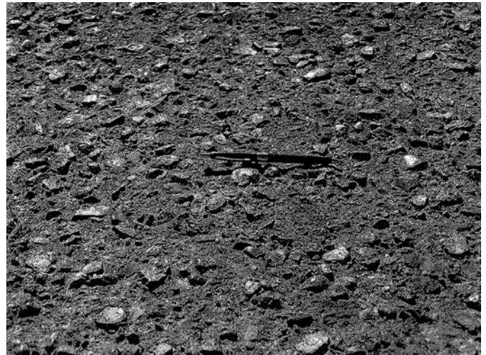
FIG. X1.81 High-Severity Weathering (Surface Wear)
