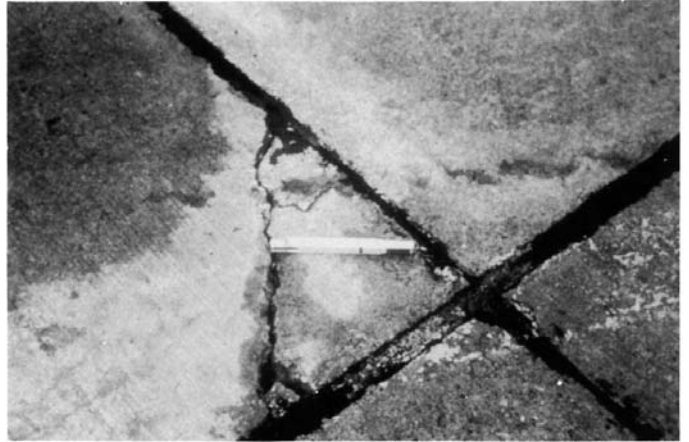
FIG. X2.70 Medium-Severity Corner Spall
