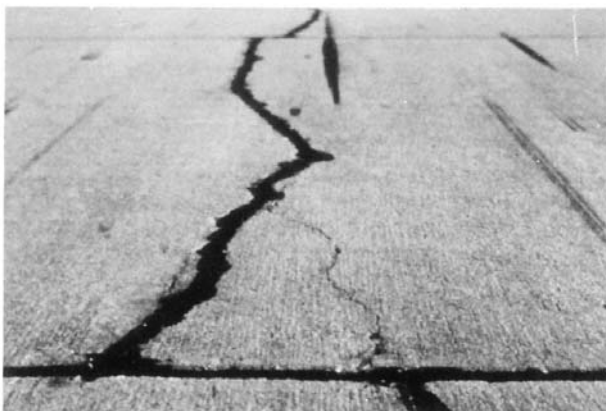
FIG. X2.16 High-Severity Longitudinal Cracks
