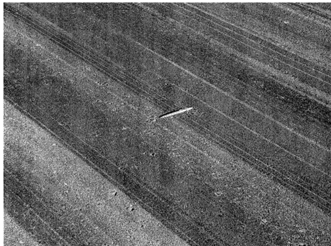
FIG. X1.54 Low-Severity Raveling, Dense Mix
