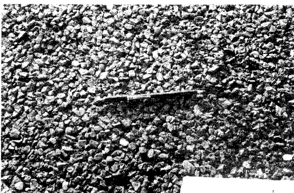
FIG. X1.64 Medium-Severity Raveling on a Porous Friction Course Surface
