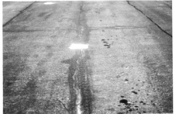
FIG. X1.40 Medium-Severity Longitudinal Crack (Note the Crack is Reflective But Not at the Joint of Slab)
