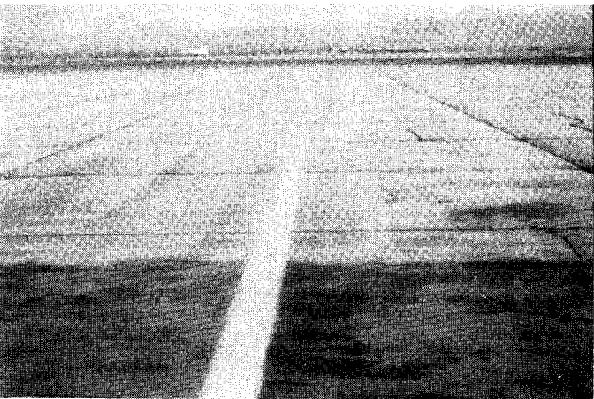
FIG. X1.30 Low-Severity Joint Reflection Cracking
