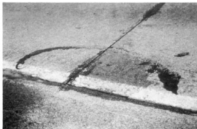
FIG. X2.39 Pumping (Note Fine Material on Surface That has Been Pumped Out Causing Corner Break)
