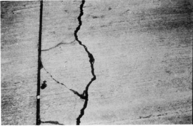
FIG. X2.64 Medium-Severity Joint Spall
