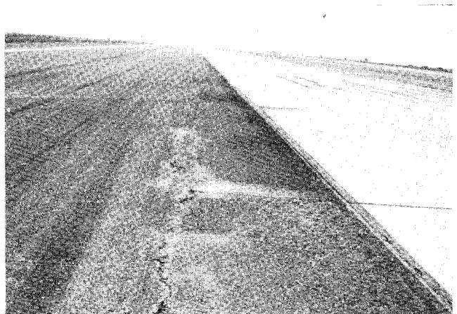
FIG. X1.41 Medium-Severity Longitudinal Crack
