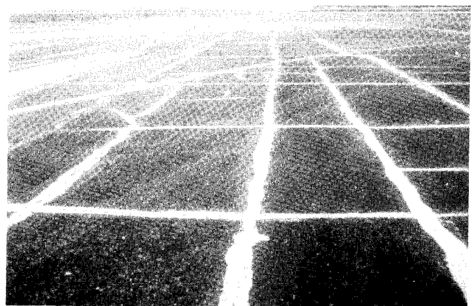
FIG. X1.13 Low-Severity Block Cracking, Filled Cracks
