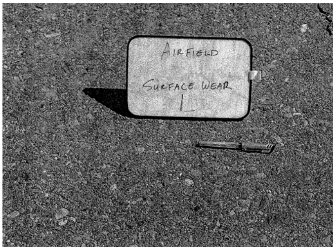
FIG. X1.79 Low-Severity Weathering (Surface Wear)
