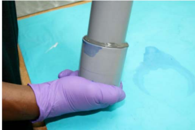
FIG. 15 Insert the pipe to the socket bottom, hold for an adequate length of time to avoid push out, and verify that there is a continuous bead of solvent cement around the entrance of the socket
